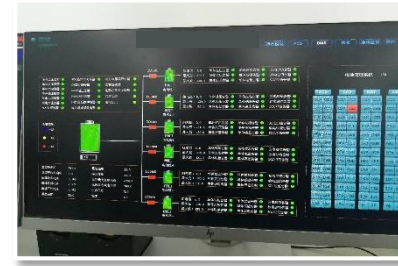
ESS project in China System efficiency < 80%
