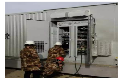
ESS project in China, experts need to manually inspect all modules in the plant
