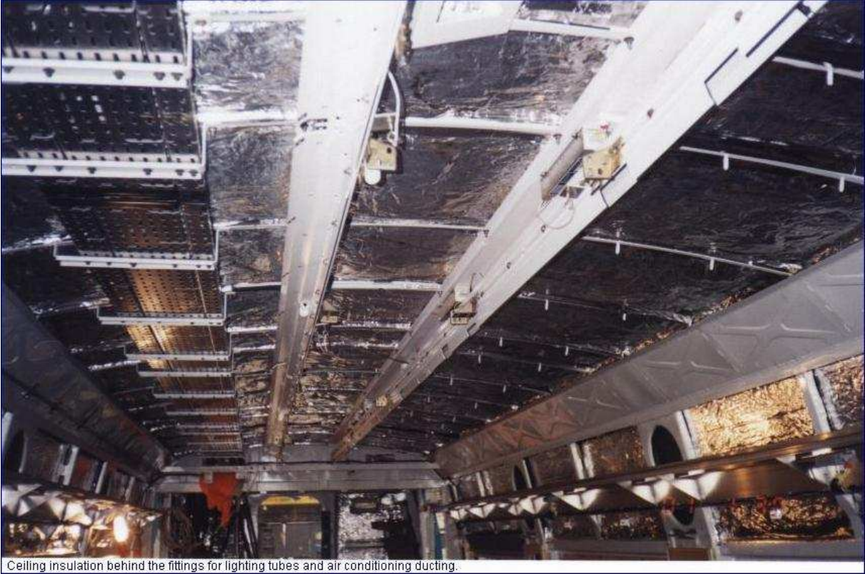
Ceiling insulation behind the fittings for lighting tubes and air conditioning ducting.
