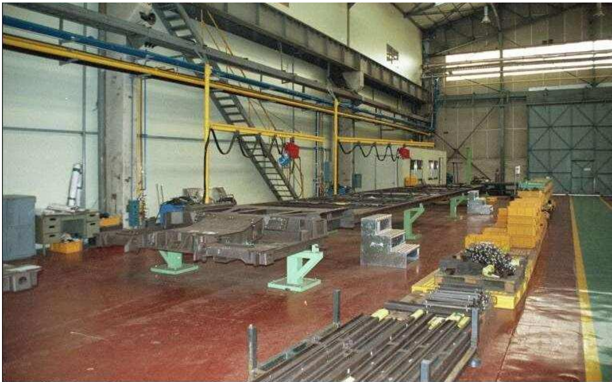
For the next steps it is still inverted but more sections are to be welded in place.
