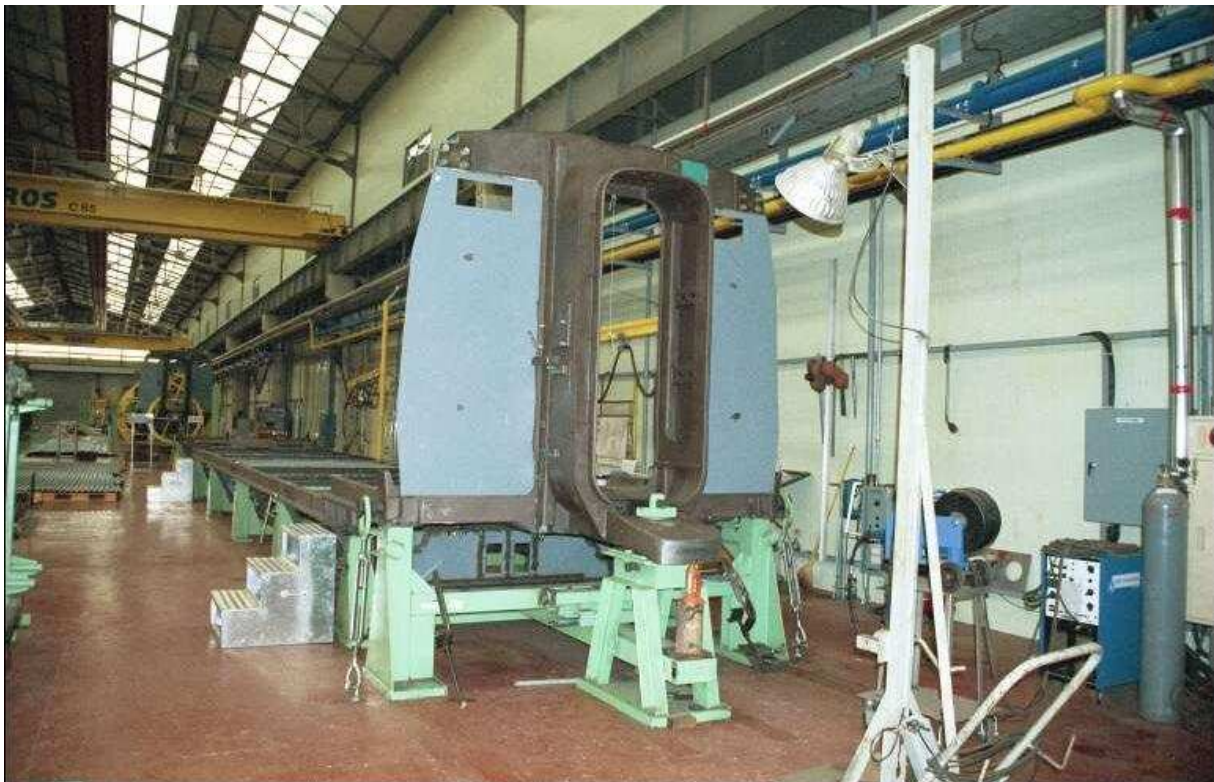
The underframe has been turned to its normal position and the car end has been welded on.
