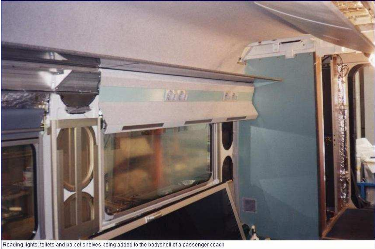
Reading lights, toilets and parcel shelves being added to the bodyshell of a passenger coach
