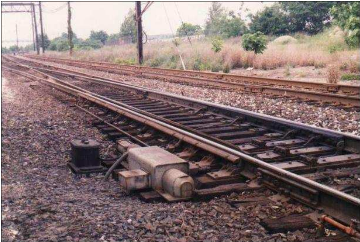
US turnout showing the electro-pneumatic motor to operate the switch blades and the point heater tube alongside the stock rail. Heaters are invaluable in cold weather conditions and are widely used. Turnout motors are usually electric but electro-pneumatic motors are seen in the US and are standard equipment for London Underground.
