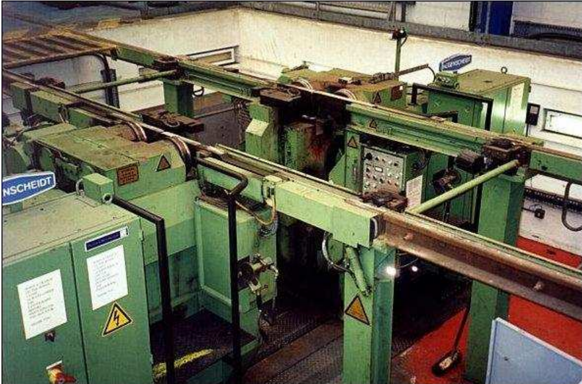
An underfloor wheel lathe for multiple unit rolling stock built into the floor of a depot. The train is pulled or pushed slowly onto the machine so that it can be stopped and positioned exactly as required. The rails under the wheels are removed and the wheels connected to a drive system. The profile of the wheel is set by the machine operator and the wheels are driven round by the machine while the new profile is cut by the fixed tool. Some machines use a milling process instead of cutting.
