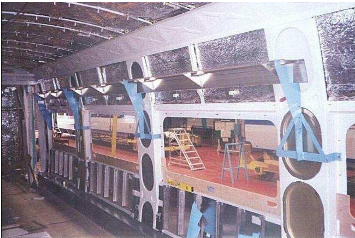
Interior of TGV trailer showing the jigs used to support the luggage racks during fitting. Note also the sound deadening material in the walls and ceiling.
