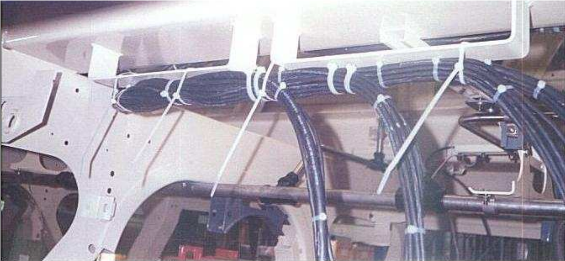
Underside of TGV car showing cable bundles fastened to the body with tie wraps. These are assembled elsewhere and are pulled through on the car.
