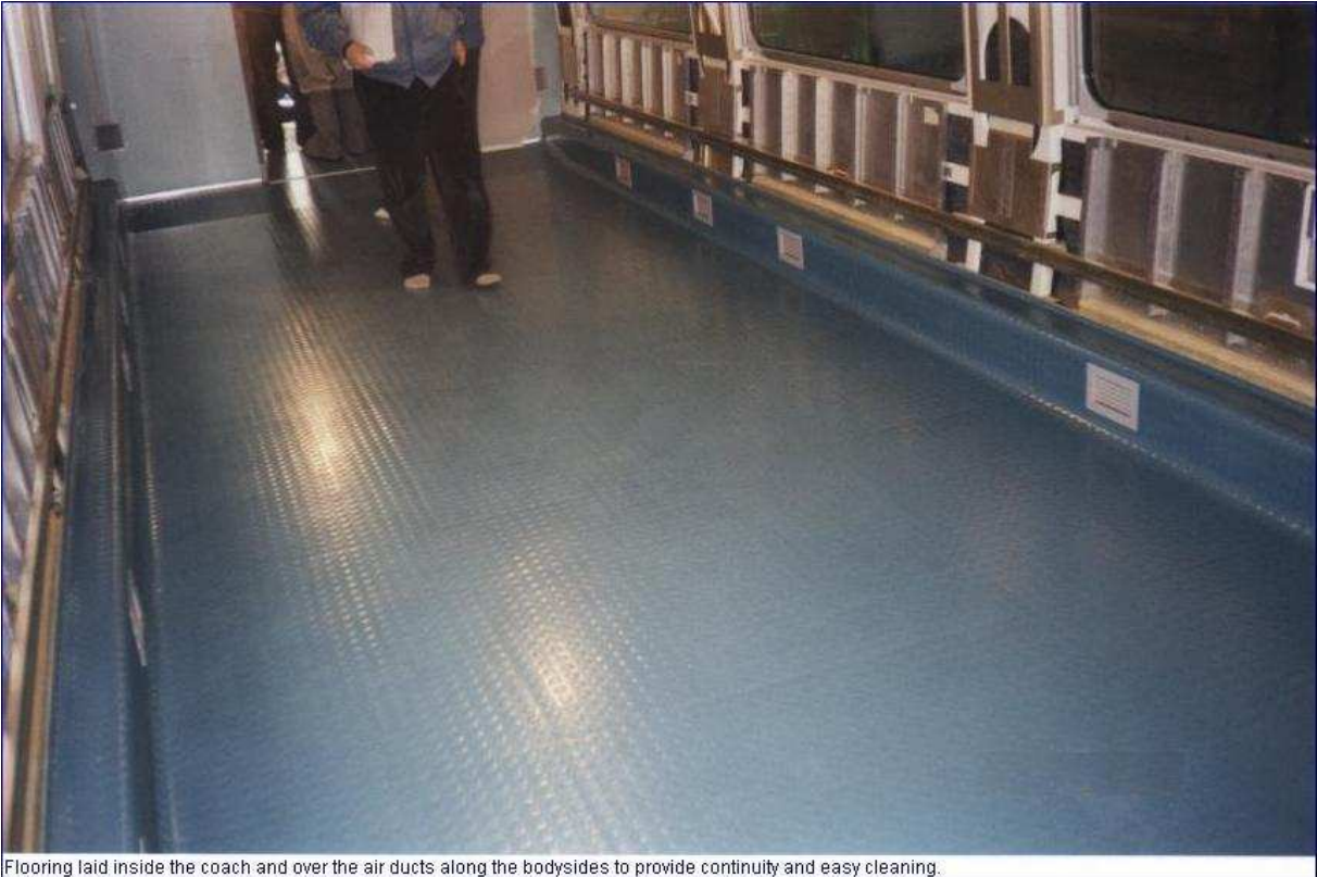
Flooring laid inside the coach and over the air ducts along the bodysides to provide continuity and easy cleaning.
