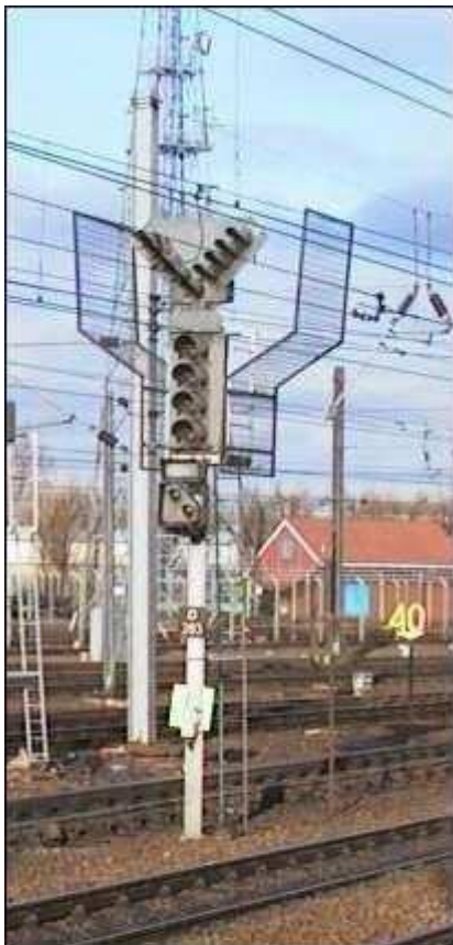
Standard UK 4-aspect junction signal. The signal can show three routes: Ahead, Diverging Left and Diverging Right. The rows of five white lights are located in the angled arms above the main signal head. Note the wire screens to protect staff from contact with the electrified overhead lines.
